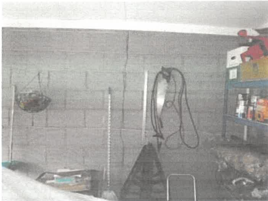
Photograph 4 – Worst of cracking to rear of LHS gable wall
