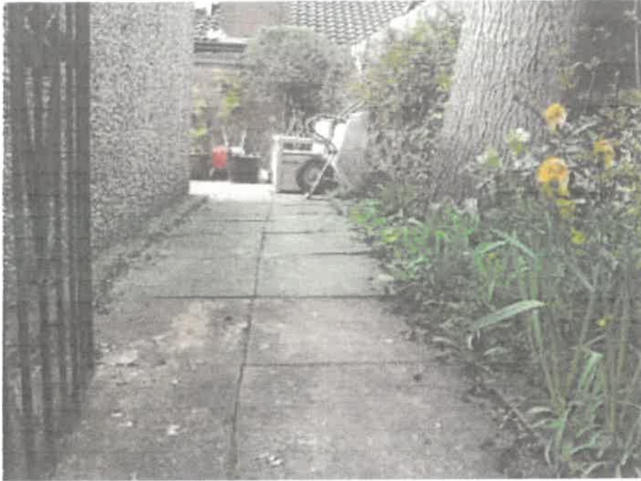
Photograph 12 – Raised slabs near tree trunk
