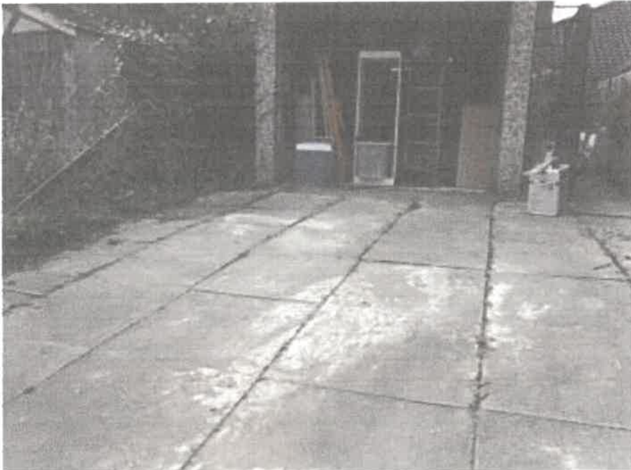
Photograph 11 – Slightly uneven slabs to front of garage
