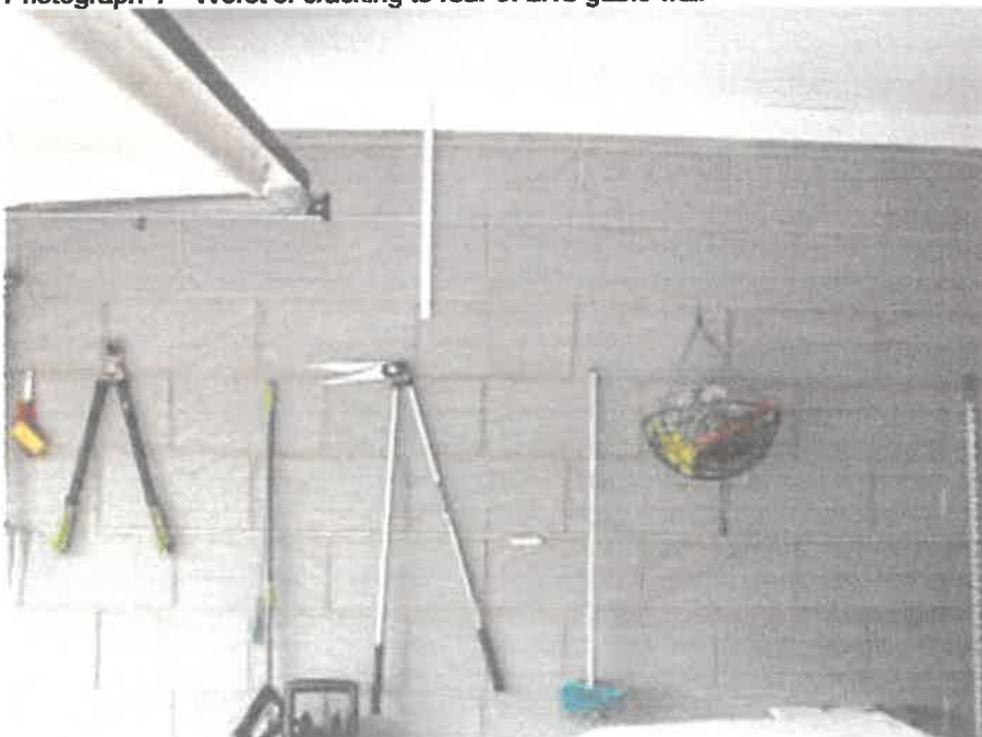
Photograph 5 – Hairline cracking to middle of LHS gable wall
