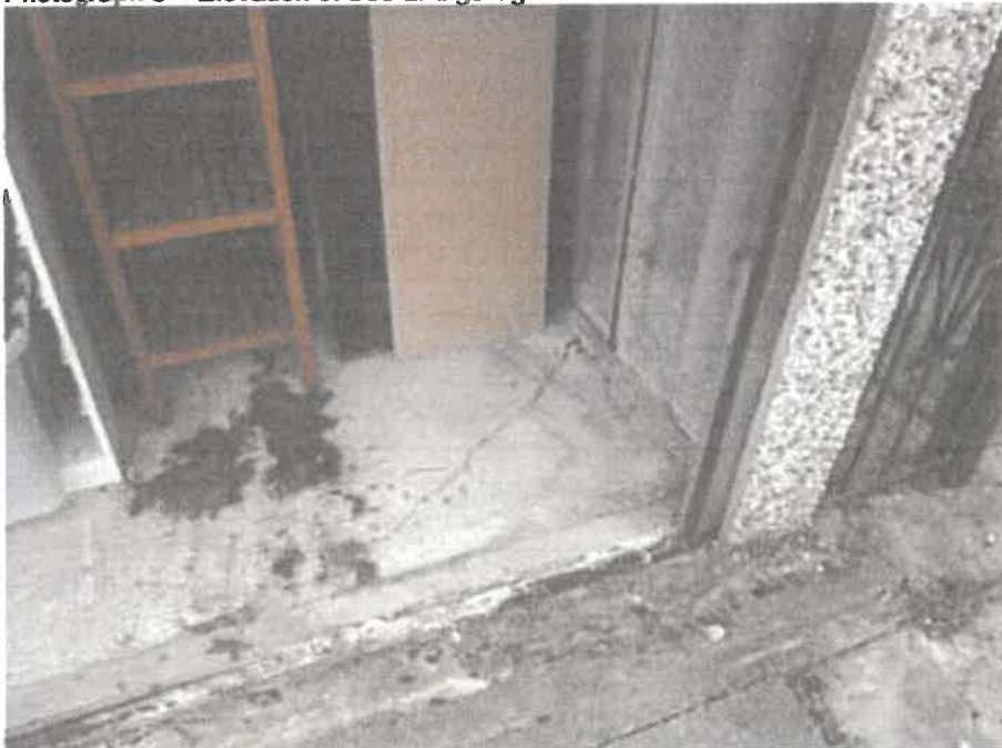
Photograph 9 – Cracking to front of garage slab
